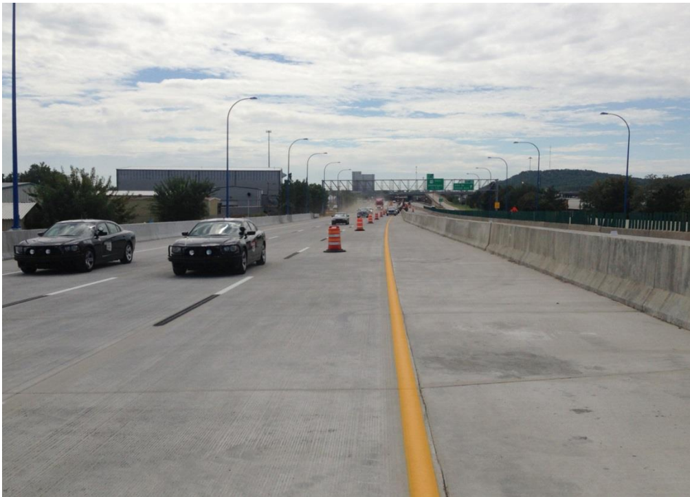
Photo 2 - The first traffic is allowed onto the new eastbound I-244 bridge over the Arkansas River in Tulsa early Monday afternoon. The eastbound bridge had been closed to traffic since the summer of 2013 as part of a $41 million replacement project. Overall completion is scheduled for spring 2015.
